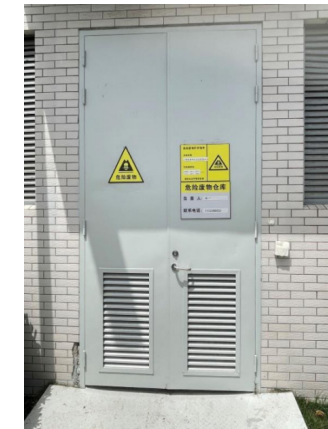
Hazardous Waste Warehouse (Shanghai Sieyuan High Voltage)
