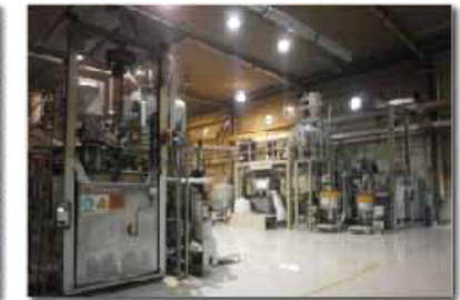
Hübers vacuum mixing epoxy casting equipment*2 sets
