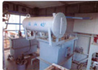
DKSC-1600/10.5-1100/0.4; XHDCZ-500/10.5 接地消弧成套装置在土库曼斯坦南约洛坦气田项目运行 DKSC-1600/10.5-1100/0.4; XHDCZ-500/10.5 complete set of arc suppression grounding apparatus is running in Turkmenistan's South Yokolan gas field
