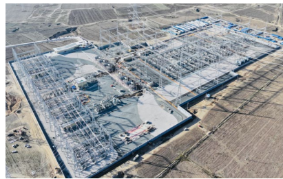
Renewable Energy Convergence Stations
