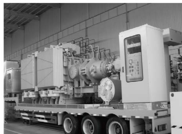
China State Grid-Fujian mobile substation project
