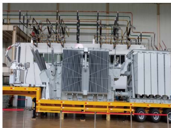
China Southern Power Grid-mobile substation project
