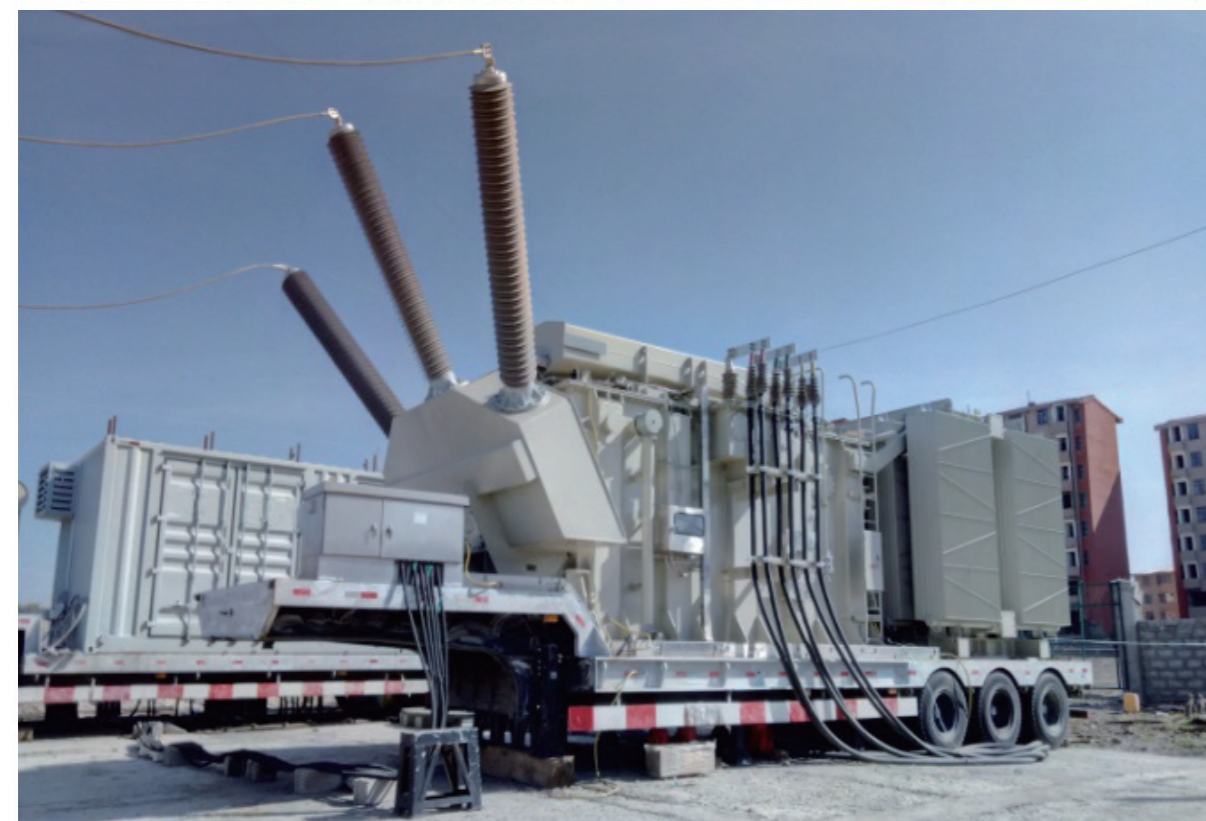
Ethiopia mobile substation project
