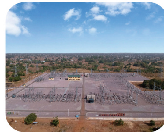
330kV Substation EPC Project, Bolgatanga, Ghana
